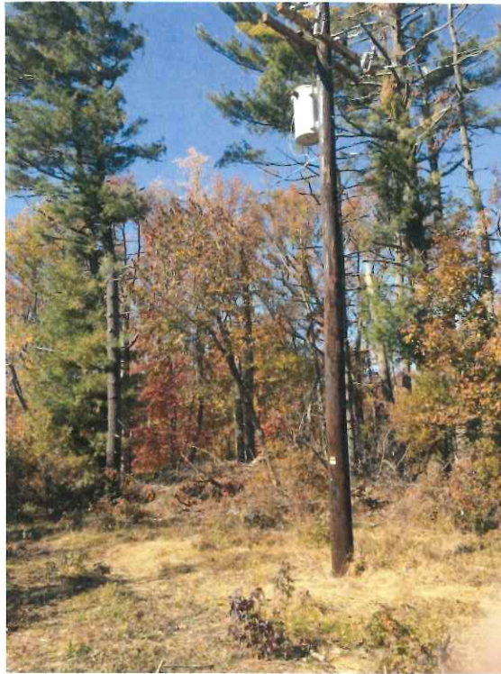
Photo 11: Pole-mounted transformer in central portion of property
