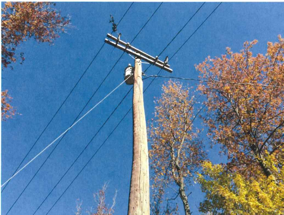
Photo 16: Pole-mounted transformer near A-Line road in western portion of Property.
