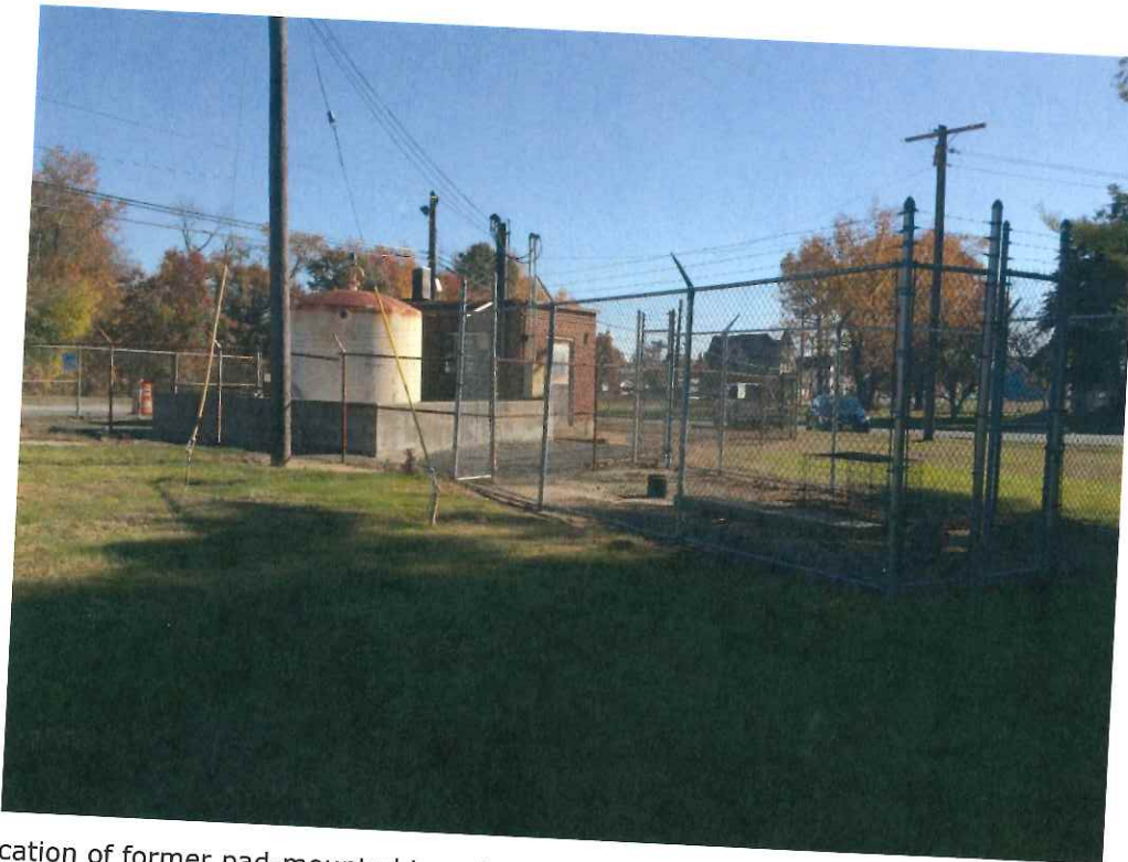
Photo 27: Former caustic AST and concrete containment adjacent to treatment building. Three pole-mounted transformers in background.
