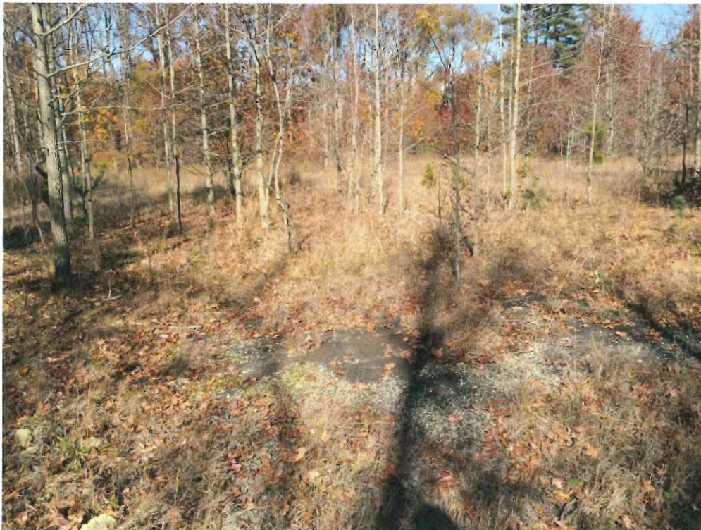
Photo 18: Old pavement in the west central portion of the property, with trees growing through degraded asphalt.
