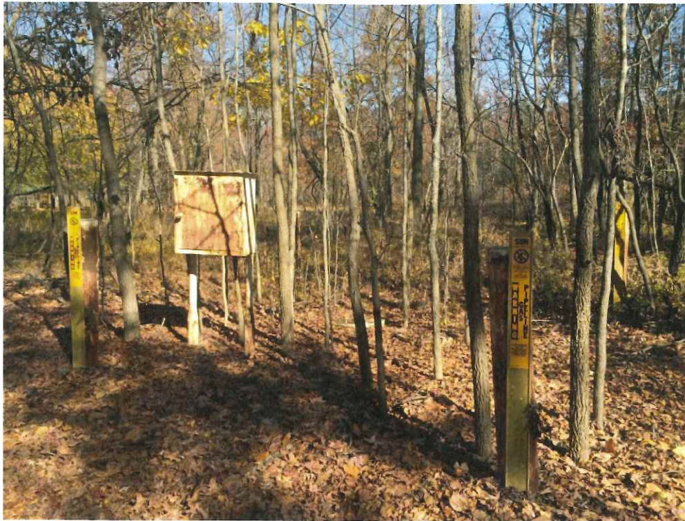
Photo 3: Sun gas pipeline markers, controls, and valve pits east of A-Line Road on the west side of the property.
